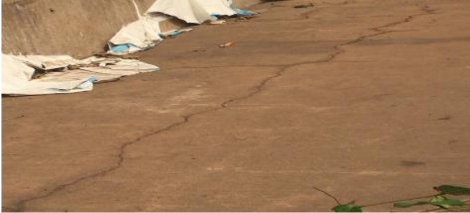
Plate 17 Cracks at walkway of the bridge on Ayingba - Abuja approach
