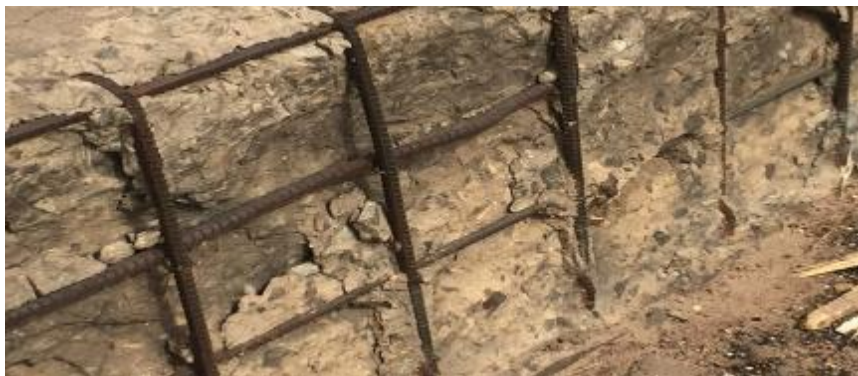
Plate 19 Concrete spalling on the pedestrian walkway protector.
