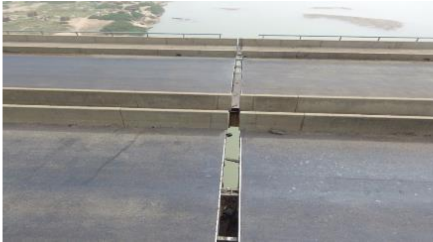
Plate 23 Drone image showing missing expansion joint cover of Itope Bridge.
