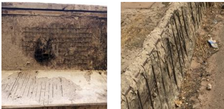
Plate 7 Corrosion of reinforcement bars at the soffit of deck.
