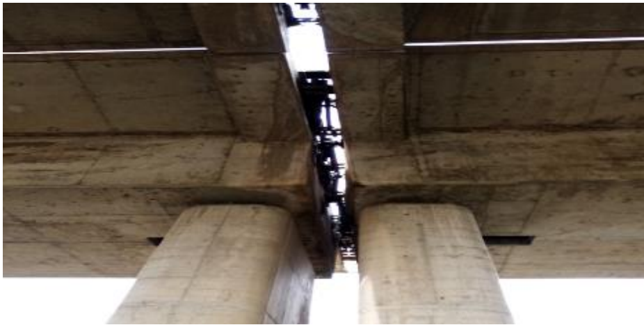
Plate 27 Image showing opening of expansion joint from the below the deck.
