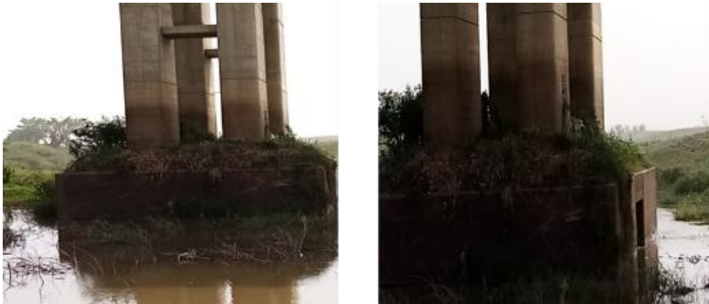
Plate 9 Scouring action exposing the pile cap No 2
