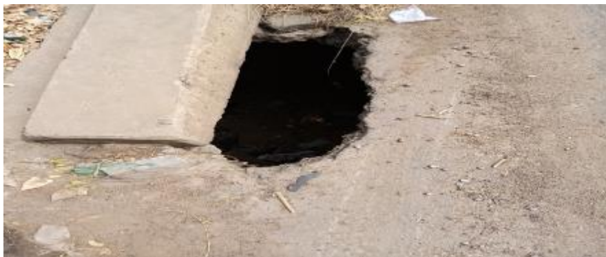
Plate 11 Erosion action exposing part of Abuja approach Abutment
