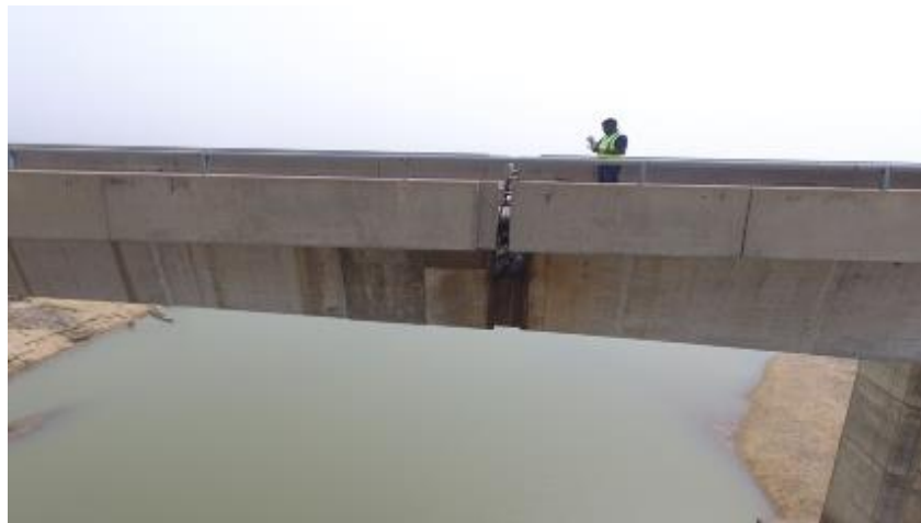
Plate 24 Drone image Showing missing expansion joint cover of Itope bridge
