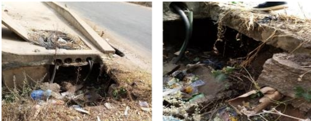
Plate 10 Erosion action exposing part of Abuja approach Abutment
