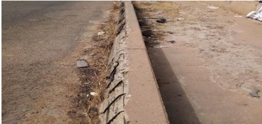
Plate 20 Spalling observed on pedestrian walkway section.
