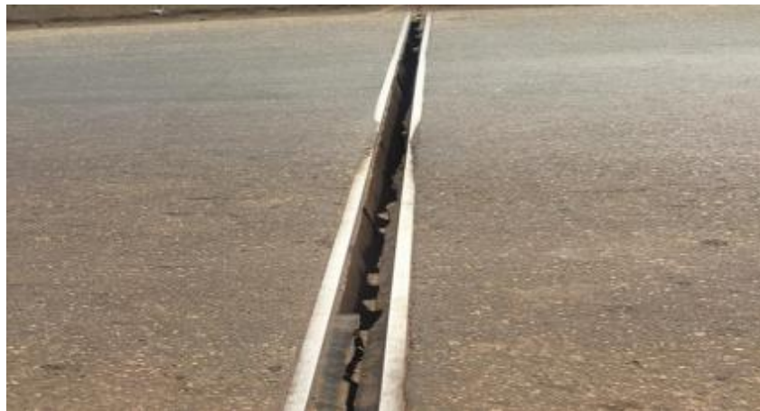
Plate 22 First expansion joint from Ayingba Approach with damaged elastomeric seal
