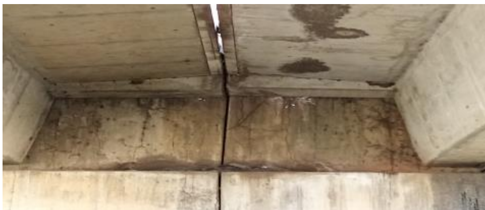
Plate 16 Minor cracks at the abutment of Abuja-Ayingba approach
