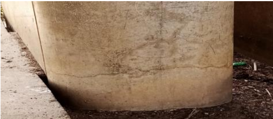
Plate 18 Crack identified on the pier foot of the Itope Bridge.
