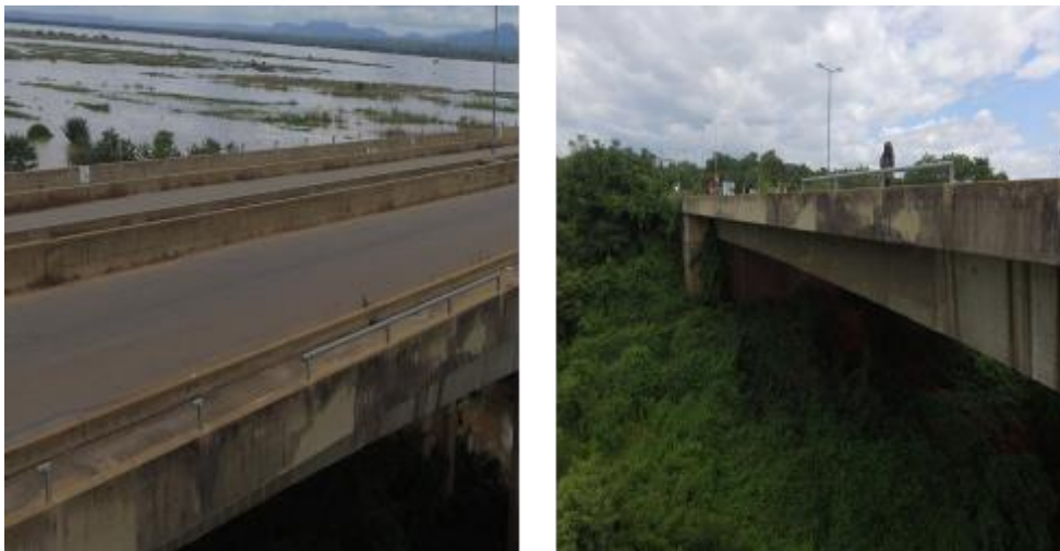
Plate 24 Image showing missing handrails.
