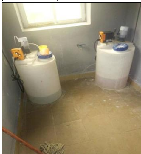
Figure 2c chemical treatment unit
