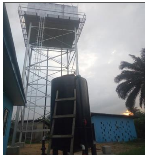
Figure 2d Pressure Filter and overhead tank
