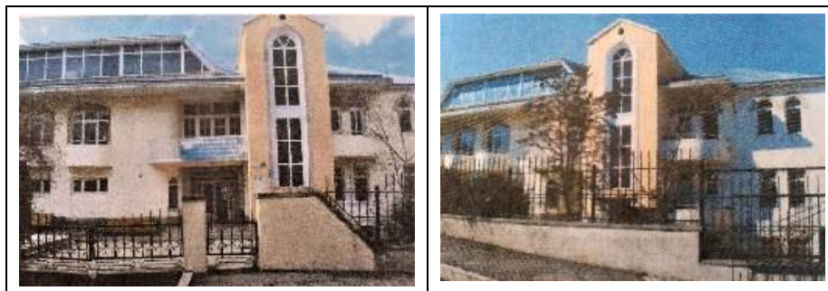
Figure 4 Views of the existing 2-story building with stone bearing walls to be retrofitted by base isolation
