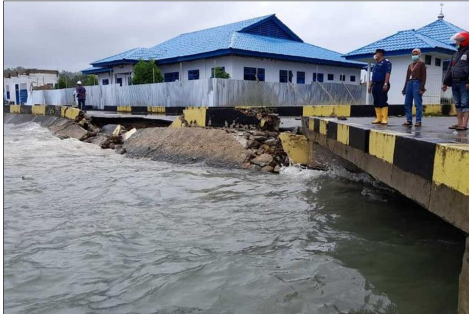
Figure 1 Conditions in the Tulehu Harbor area, Salahutu District, Central Maluku Regency, were damaged by tidal waves and floods
