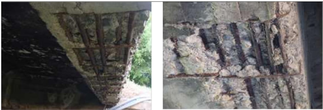
Figure 5 Concrete spalling due to reinforcement steel corrosion
