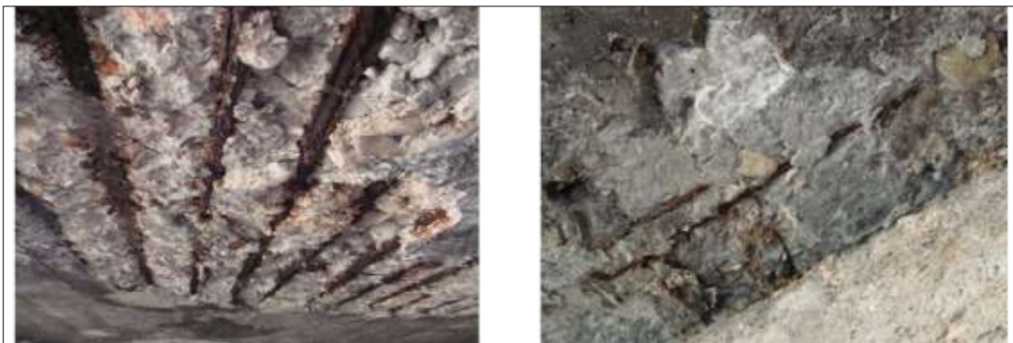
Figure 1 Concrete carbonation and steel corrosion on a bridge deck
