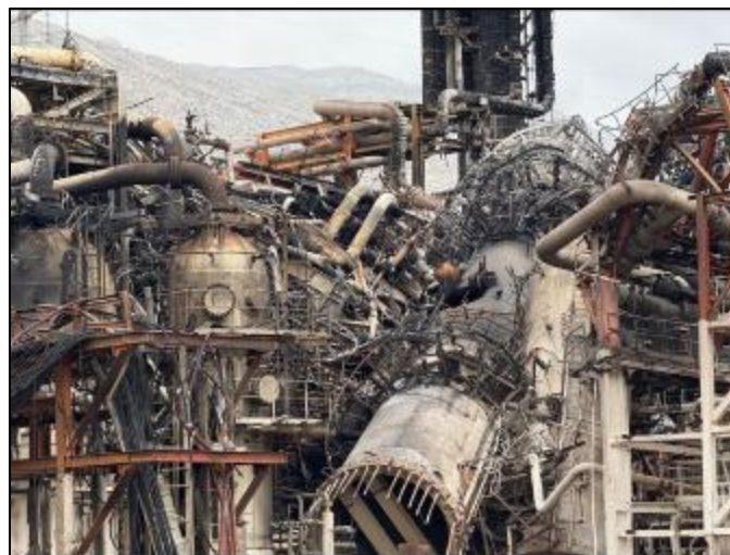
Figure 2 Field damage condition requiring stationary equipment restoration assessment. (Ref. LinkedIn)
